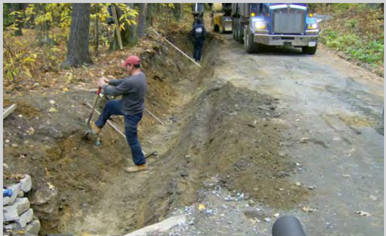
Stormwater drainage improvements to Four Mile Brook Road in Northfield were funded by Ch. 90 and a grant from Mass DEP's 319 program.
