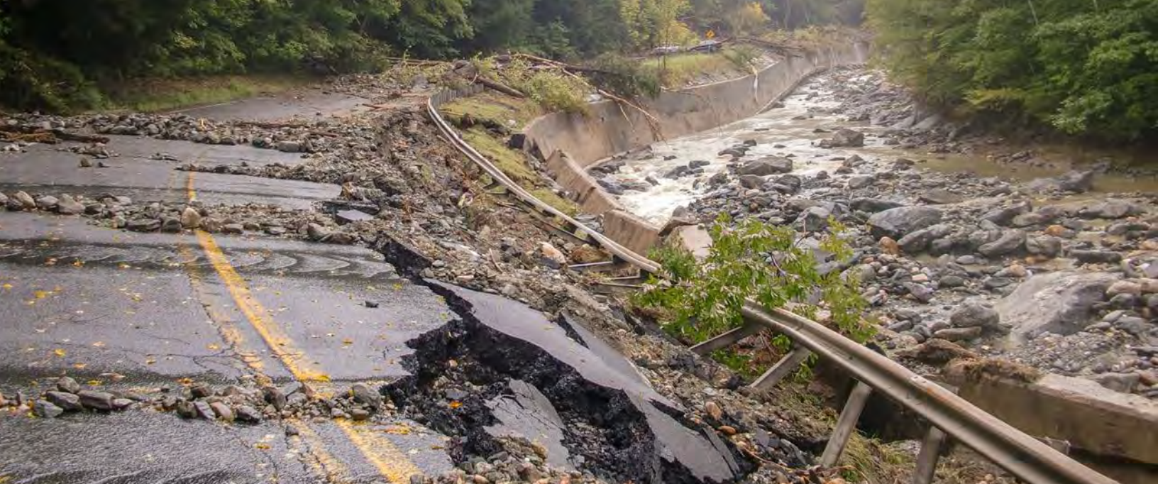
Route 2 in Charlemont was closed for three months following Tropical Storm Irene.
