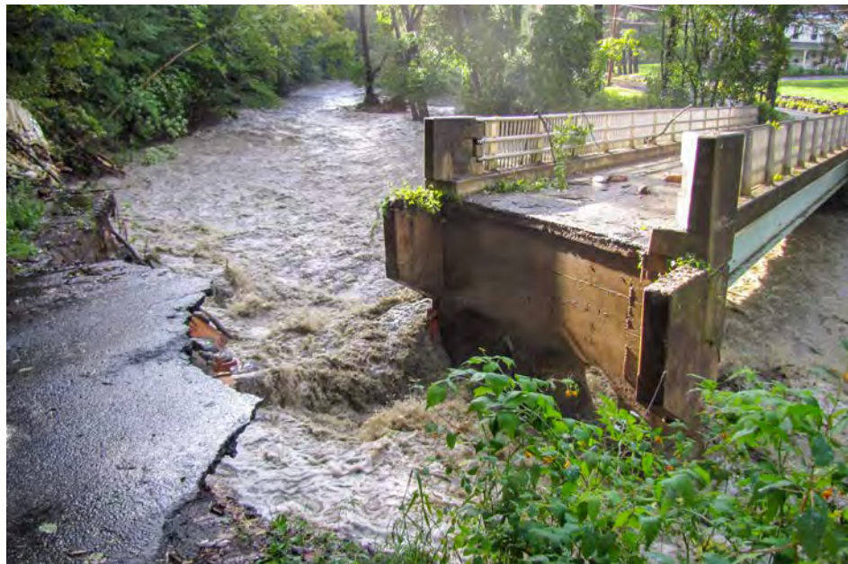
Irene's waters carried a portion of this road and bridge away on the North River in the Town of Colrain.
