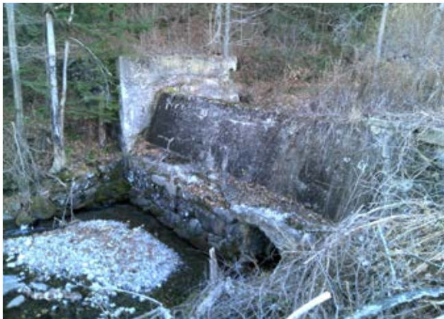
Although the dam on Foundry Brook is partially breached, it still acts as a fish barrier and hydraulic/flood barrier.
