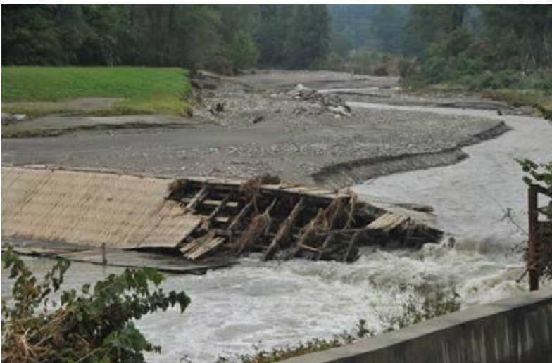
After Tropical Storm Irene, the dam was largely washed away.
