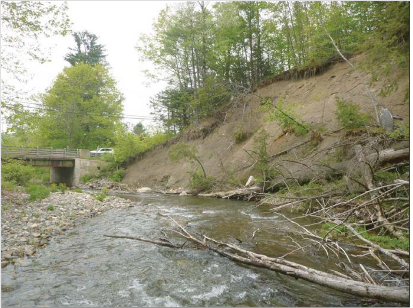
Lower Clesson Brook - photo of mass failure just upstream of Route 112 crossing on lower Clesson Brook.
